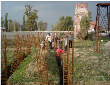
Building on Byzantine foundations / extending the Kingdom (Workers at the construction site of the Church).
